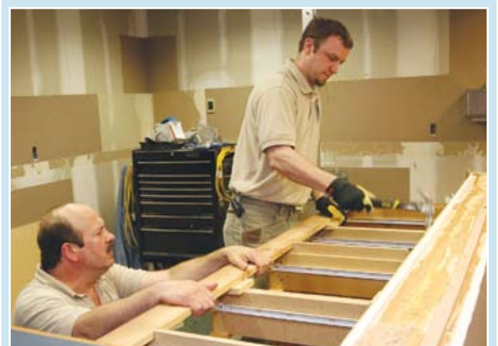
As they demolish the National Avenue Building, workers collect doors, hardware and furniture that will be reused at facilities through the system.
